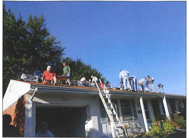
The men's Sunday School class from our church put a new roof on our house this summer. About 20 men came to help and they were finished in five hours!
